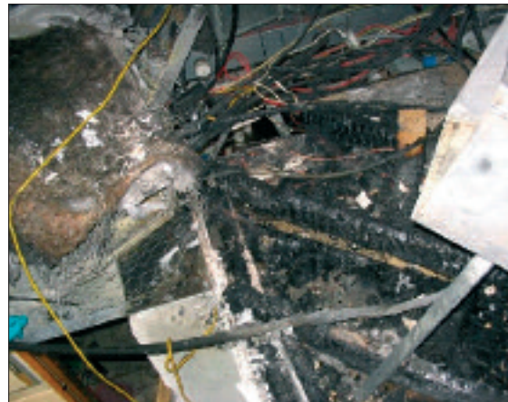
Figure 18: Station fire (courtesy of Network Rail)
